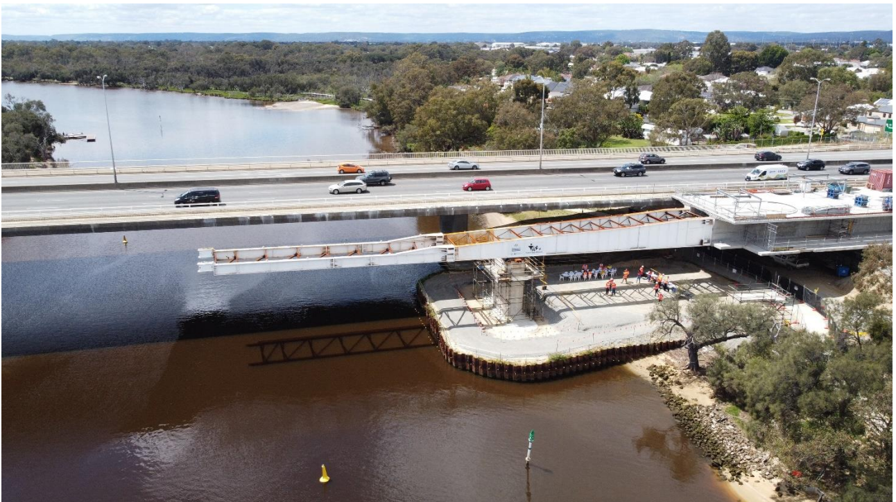
Figure 9 First launch from the southern side of the river with extended girder
