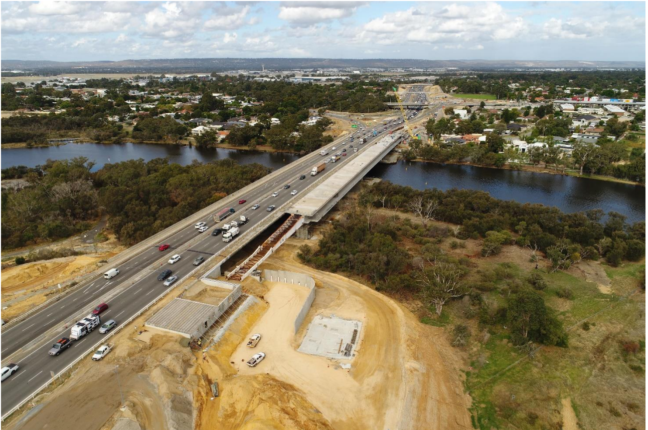
Figure 8 Drone view of completed Derbarl Yerrigan bridge launch (from the northern side)
