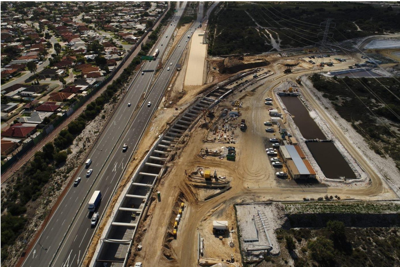
Figure 12 Aerial photo of the northern dive construction looking north, showing the threatened ecological community to the north and east of the construction site, with Tonkin Highway to the west.
